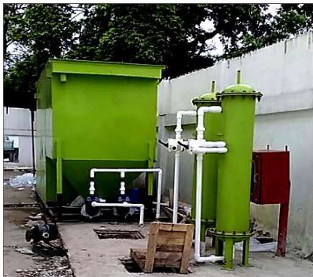
Hospital Prefabricated STP
